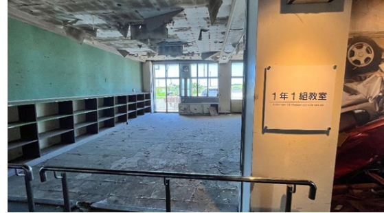
First-floor Classroom Post-Flooding
