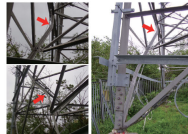
Figure1: Example of damage in Niigata Chuetsu Offshore Earthquake
